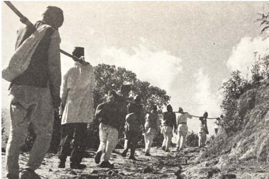
Nepalis carrying cable to ropeway towers in 1960. The entire project was built by hand.
